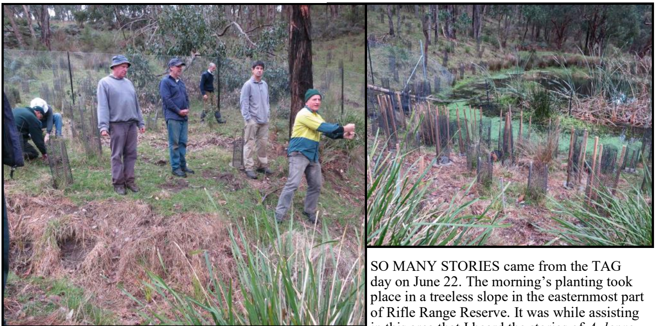
Tony demonstrates how to build a deer fence by doubling the star pickets.
