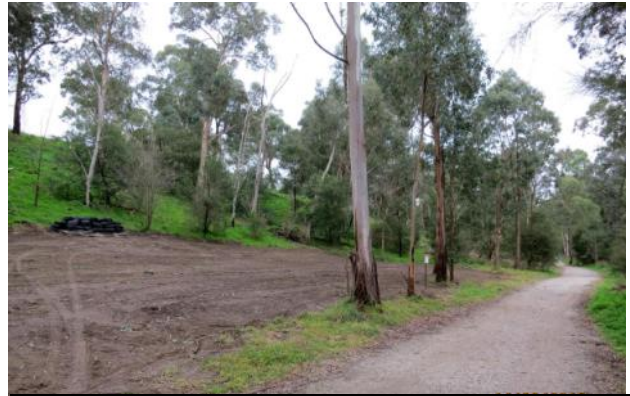
The rabbit warrens have been levelled and the ground compacted in preparations for planting.
