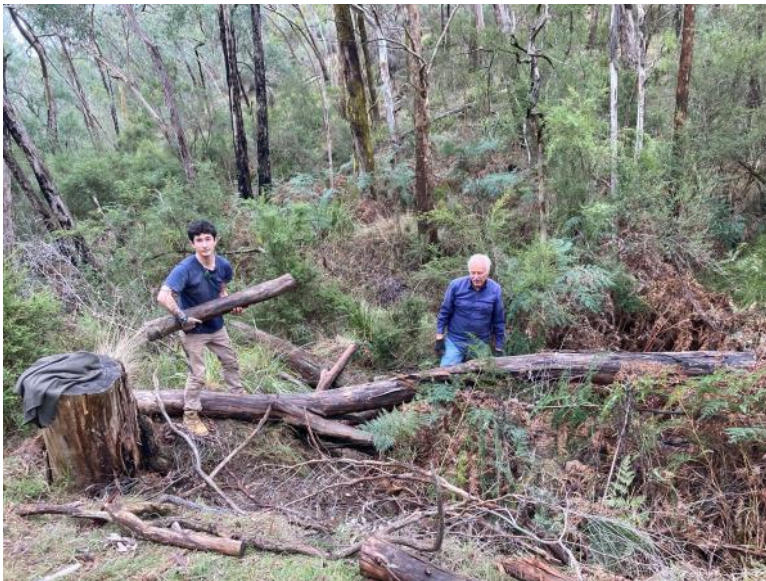
Our ACL partners ( Fritz on the right) hard at work clearing a site...
