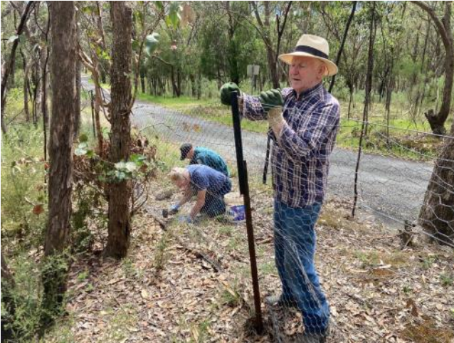
Above: Dave with Brian and Phil on fence repairs at Fiddler Fence
